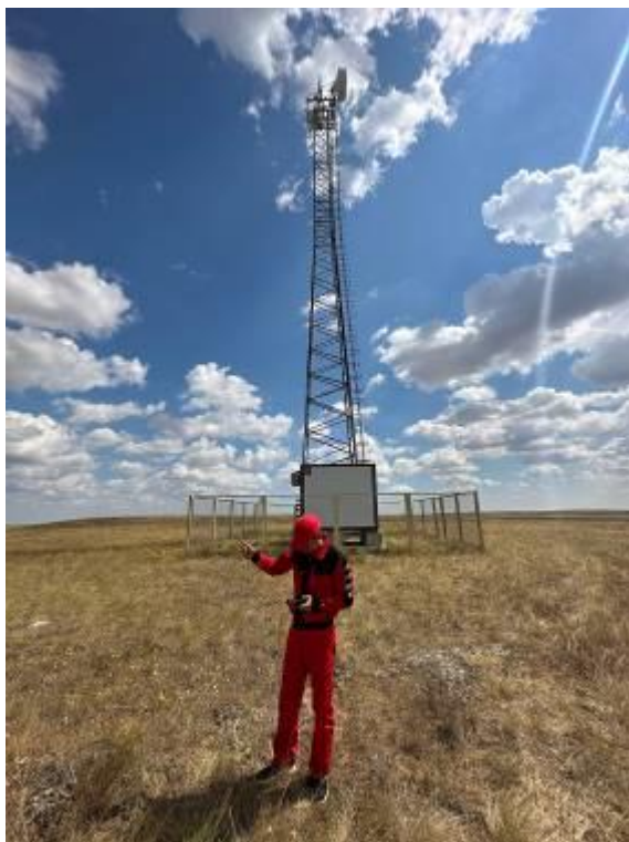
Photo 5.5. Radio transmitting devices on AMS
